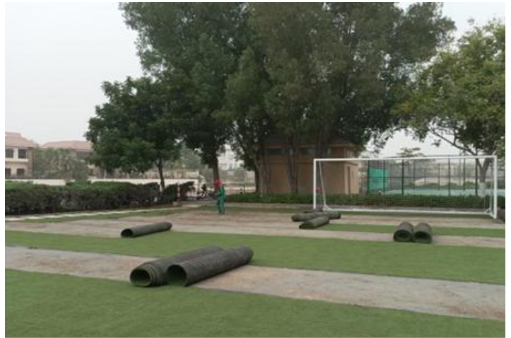
Removal of existing Astroturf & ground compaction completed; installation of new Astroturf by 29.08.2022
